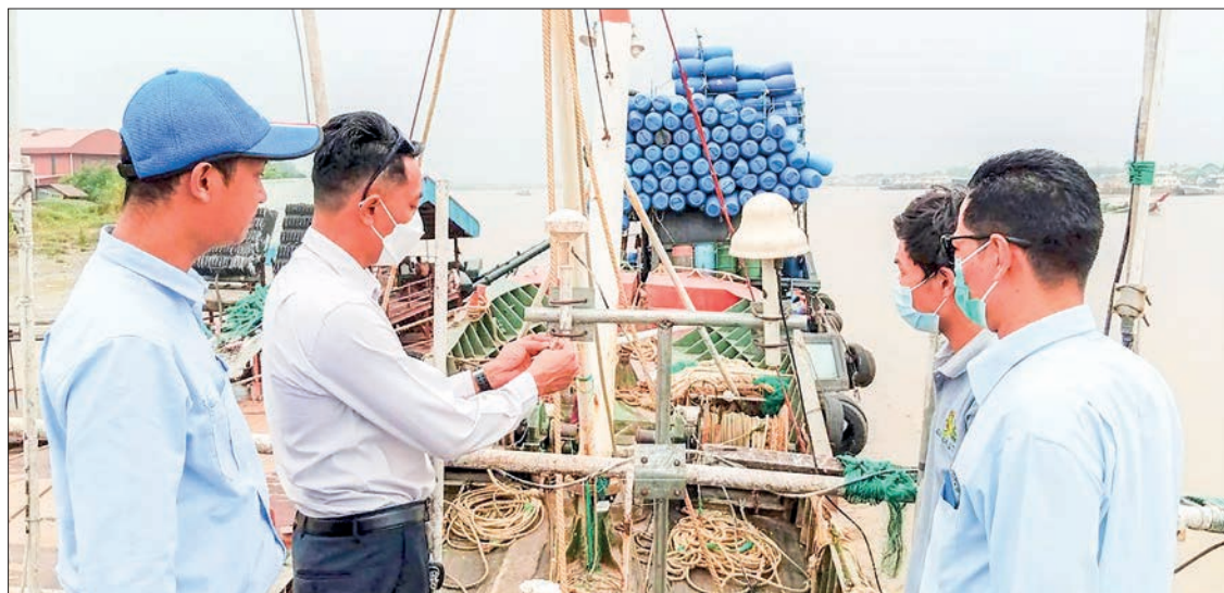
Officials install VMS system device at fishing trawler to monitor situations of fishing trawlers. PHOTO: KANU
