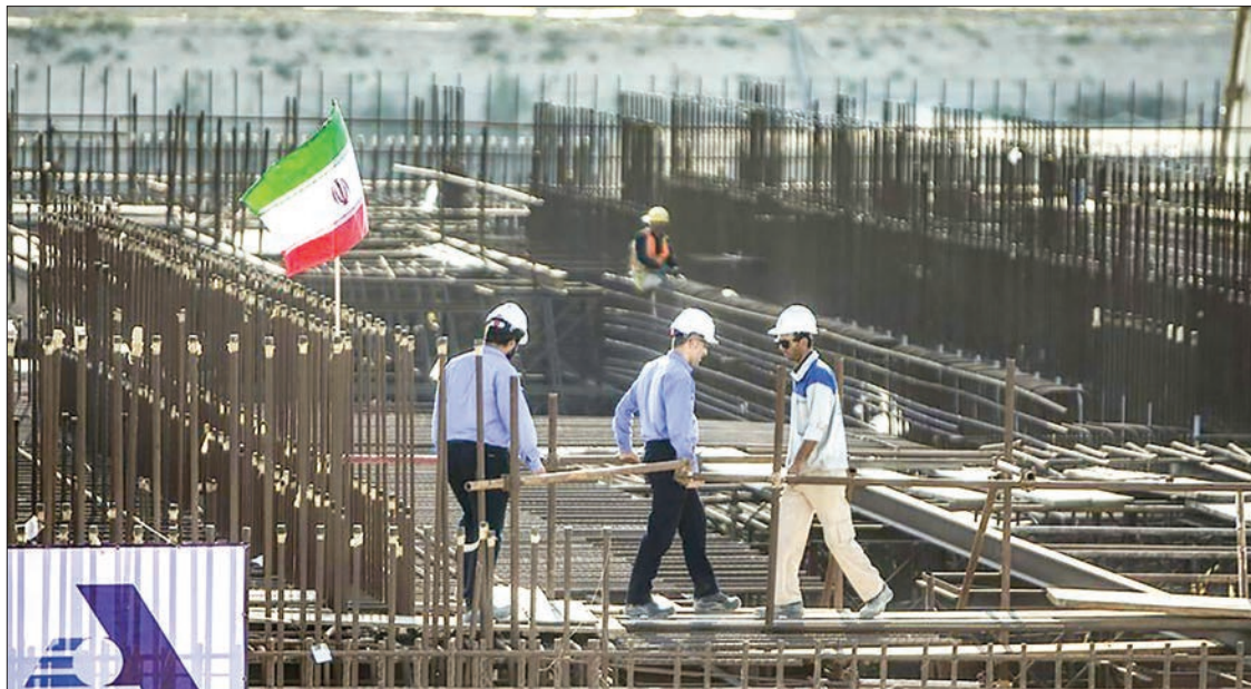
People work at the construction site of the second phase of Iran's Bushehr Nuclear Power Plant in Bushehr, southern Iran, on 10 November 2019. PHOTO: PHOTO BY AHMAD HALABISAZ/XINHUA
