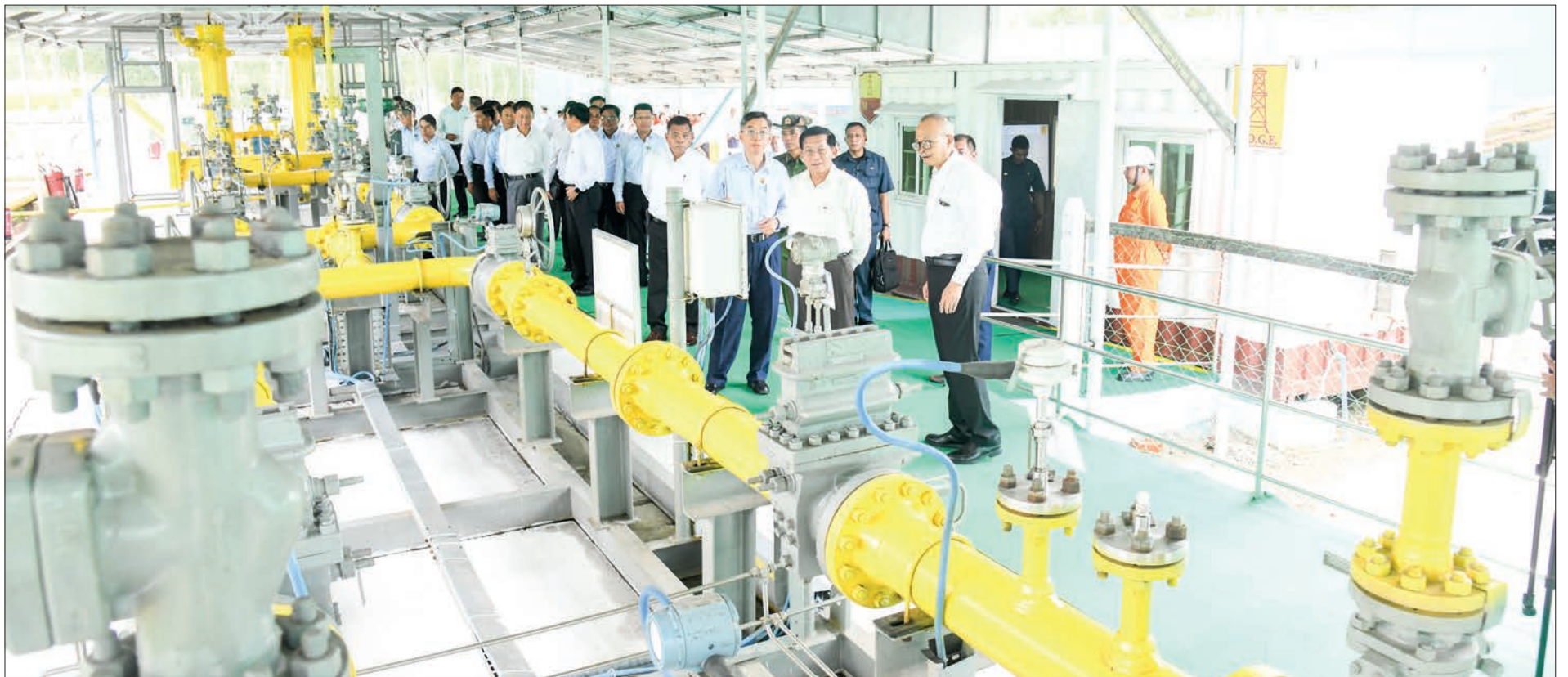
The Senior General inspects the supply of natural gas through a filtration system, pressure regulation system and metering system at the Thaboung natural gas distribution camp yesterday.
