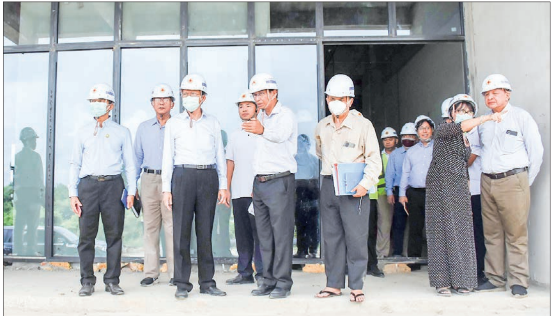
Union Minister for Health Dr Thet Khaing Win visits the ongoing construction of the China-assisted Myanmar Centre for Disease Control and Training Centre for Medical Staff (Myanmar CDC) in Nay Pyi Taw on 19 August 2023.
