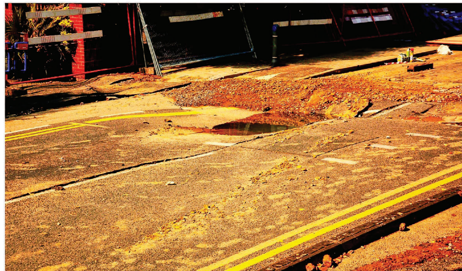
A heat wave in July 2022 caused major cracks in a roadway in Kingston upon Thames, a town in Greater London. Concrete expands in high heat, as do many other materials crucial to infrastructure and technology. Engineers and materials scientists are studying ways to manage increasing temperatures, including how to capture and reuse expended heat from machines and other devices.
