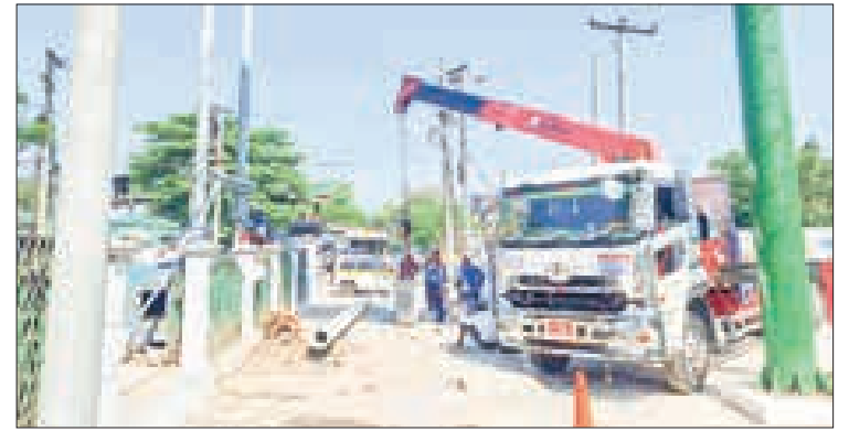
The photo shows the Yangon-Pyay Road extension during relocation and construction of power lines and transformers that are not free from the road.
