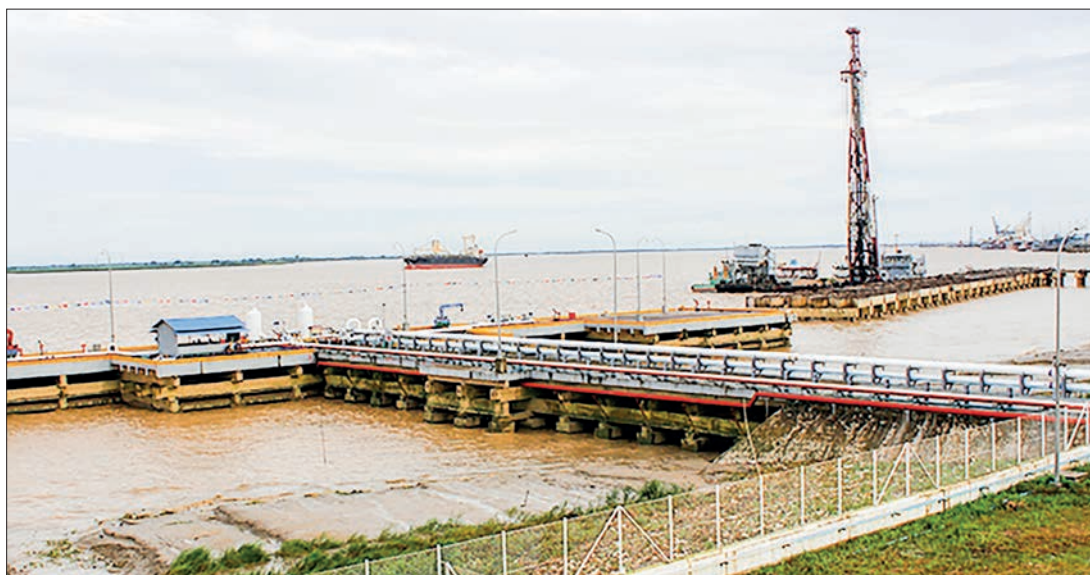
The jetty of Thilawa Port arranged to admit handling of fuel loading and unloading in July.
