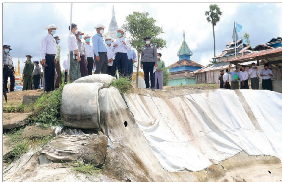
MoTC Union Minister Admiral Tin Aung San inspects the landslide protection work.
