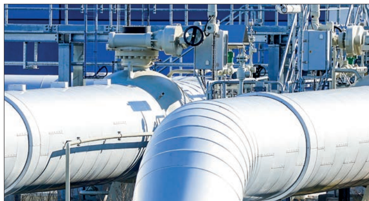
A valve wheel on pipework at the Radeland 2 compressor station for the European Gas Pipeline Link (EUGAL), a downstream pipeline for Nord Stream operated by Gascade Gastransport GmbH, in Radeland, Germany, 11 March 2022. PHOTO: CFP/CGTN/XINHUA
