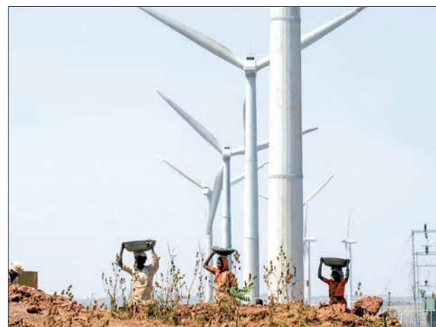
A wind farm under construction at Vankusawade in Satara district, in the western state of Maharashtra, India. PHOTO: SEBASTIAN D'SOUZA/AFP
