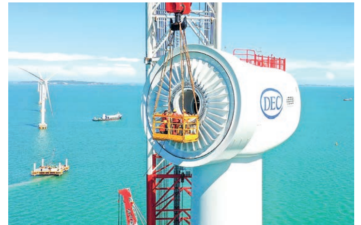
Aerial photo taken on 12 June 2020 shows workers installing an offshore wind turbine at a wind farm in Fuqing, southeast China's Fujian Province. PHOTO: LIN SHANCHUAN./XINHUA
