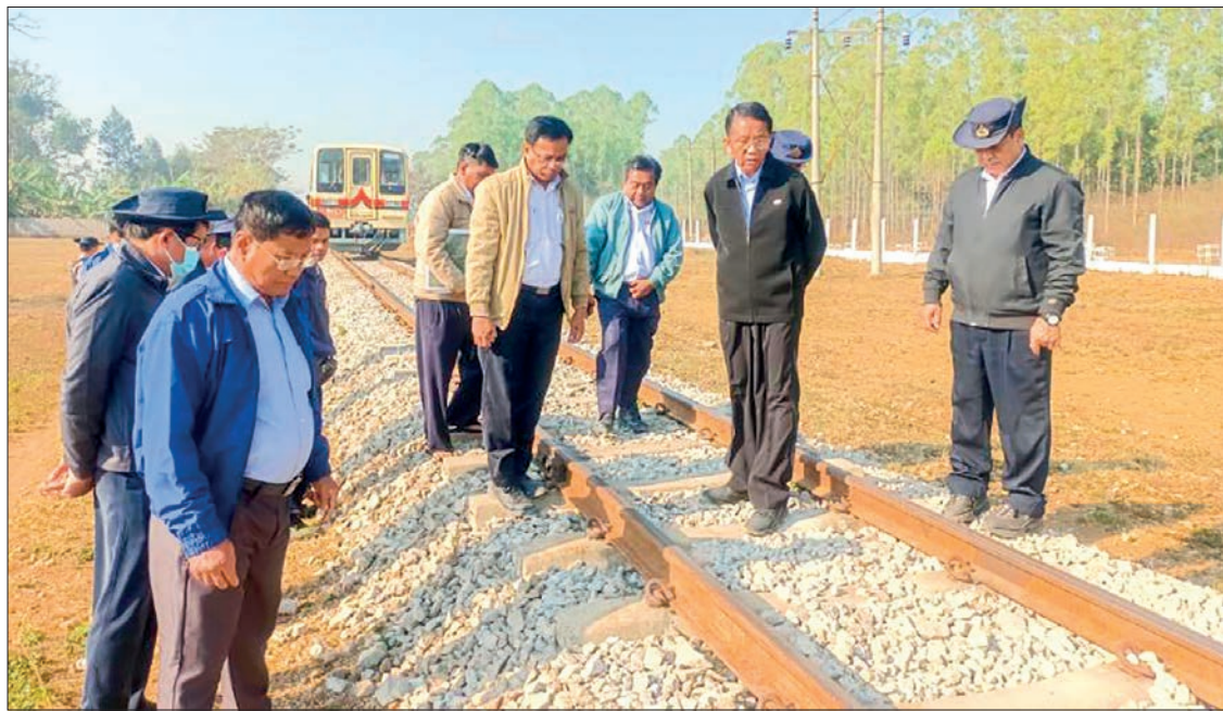
The MoTC deputy minister and party are pictured during the inspection of railway lines.
