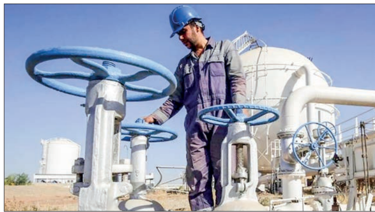
An Iraqi oil employee checks pipelines at the Bai Hassan oilfield, west of Kirkuk, 19 October 2017. PHOTO: AFP/FILE
