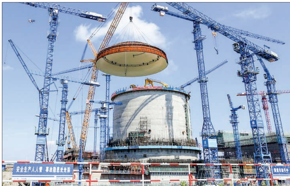
Photo taken on 23 May 2018 shows the installation site of a hemispherical dome at the No. 3 unit of Fangchenggang nuclear power station in south China's Guangxi Zhuang Autonomous Region. PHOTO: FANGCHENGGANG NUCLEAR POWER CO., LTD/ XINHUA
