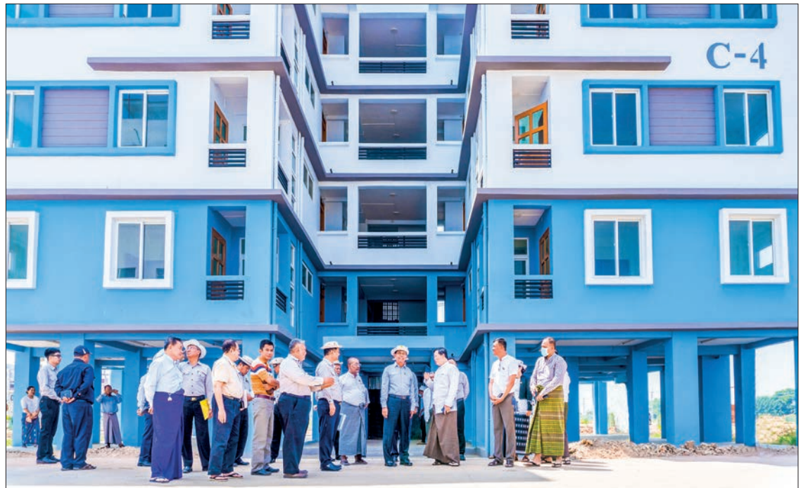
Union Minister U Myo Thant inspects the public rental housing construction project site yesterday.
