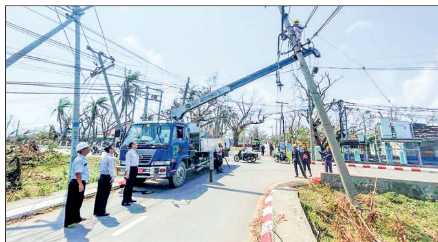
The re-erection and reinstallation of electricity poles and power cables underway in Sittway.
