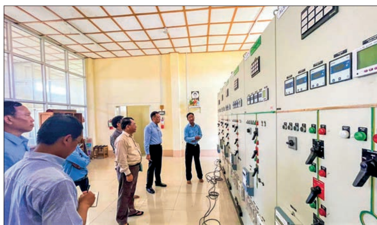
Deputy Minister for Electric Power U Aye Kyaw inspects control room of Ponnagyun main station on 21 May.
