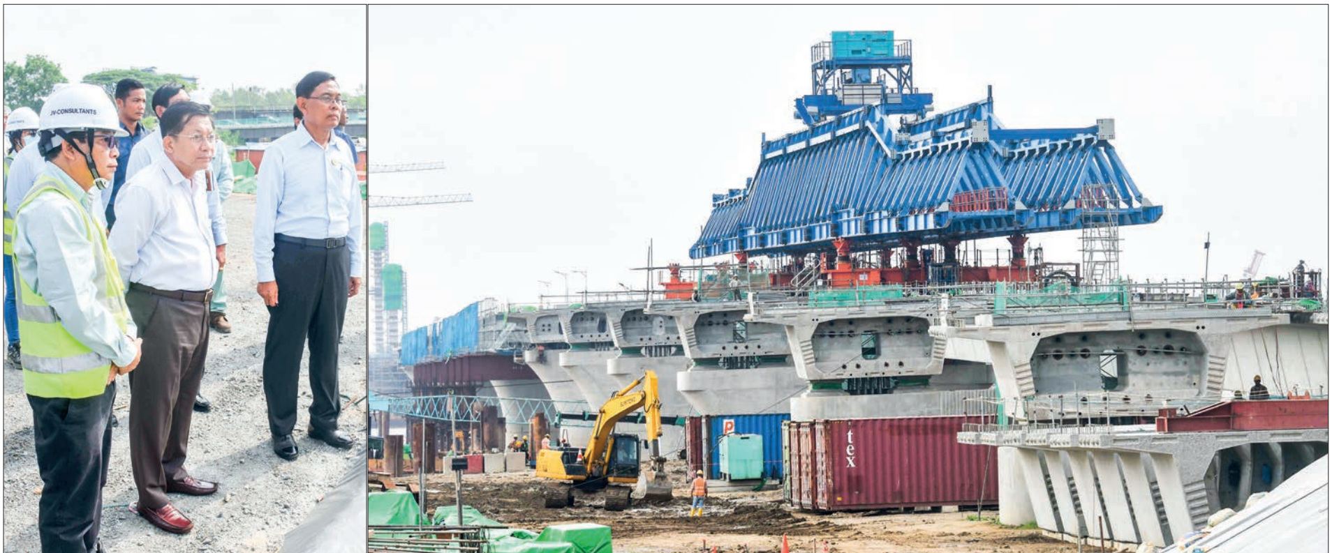
SAC Chairman Prime Minister Senior General Min Aung Hlaing inspects progress of Bago River Bridge (Thanlyin Bridge-3) in Yangon Region on 21 May.
