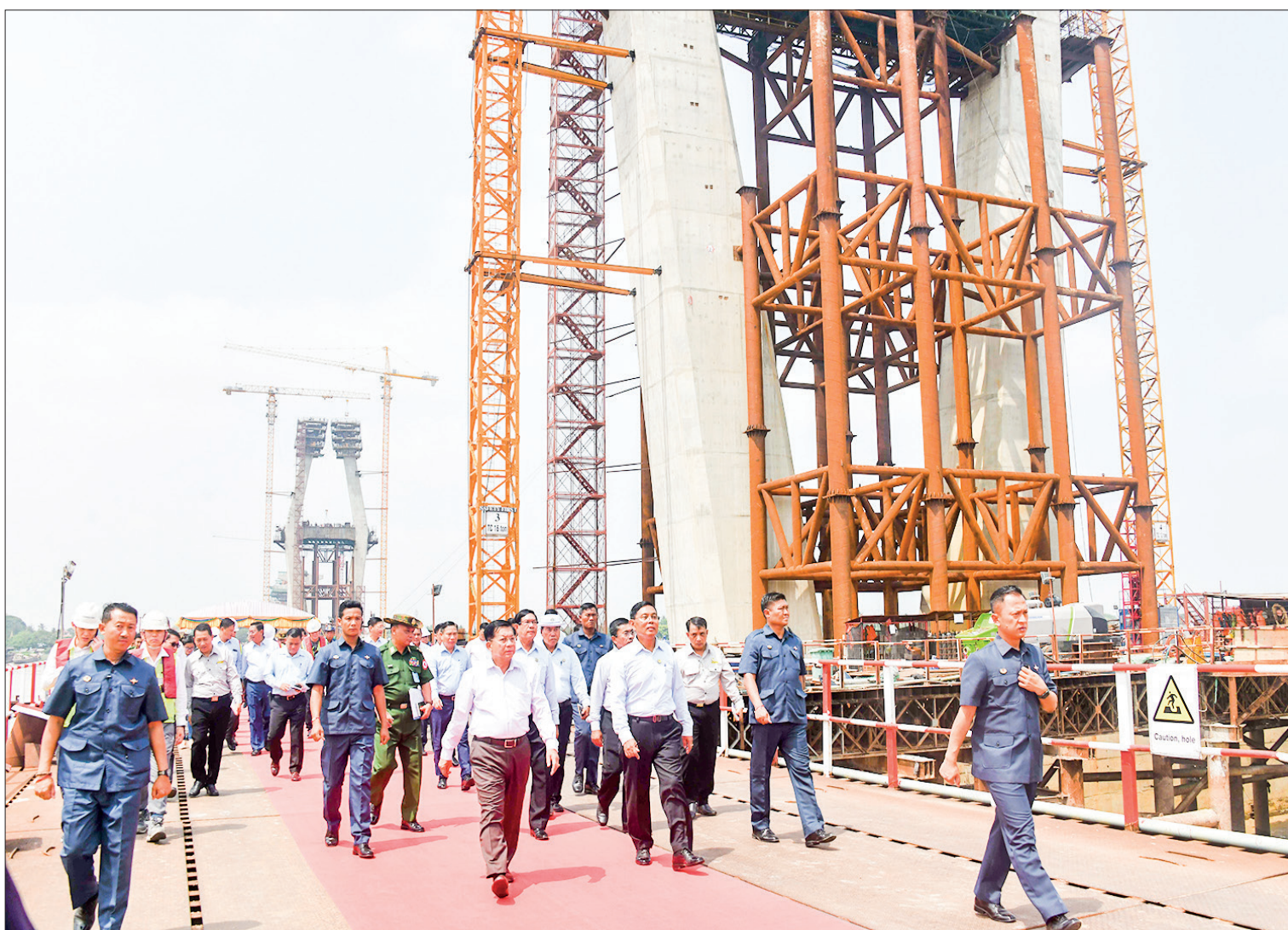
Senior General Min Aung Hlaing looks into implementation of Myanmar-Korea friendship (Dala) bridge project site on 21 May.
