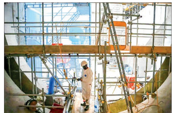
A workman wearing PPE works at the Thames Tideway tunnel building site, in west London, on 14 June 2023. PHOTO: DANIEL LEAL / AFP
