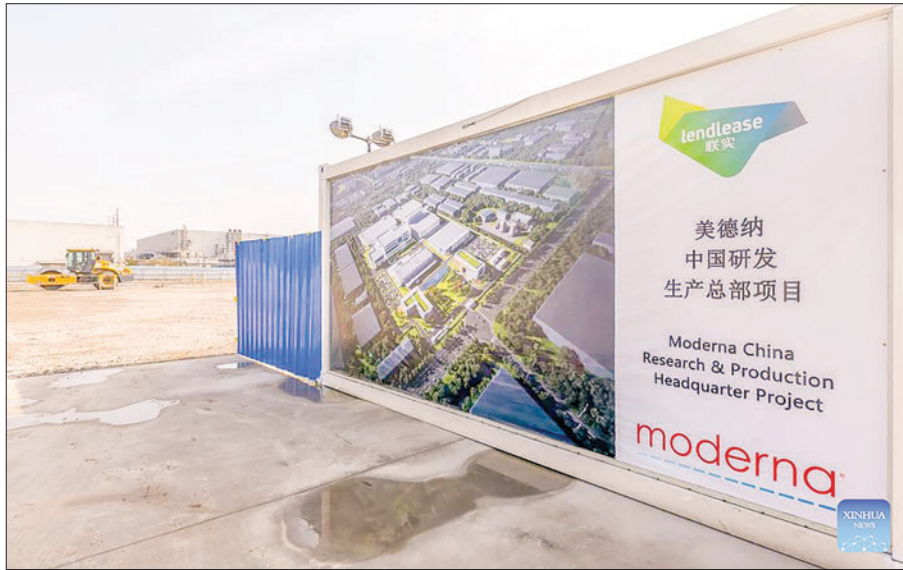
This photo taken on 20 December 2023 shows the construction site of American biotech company Moderna's pharmaceutical plant in Shanghai, east China. PHOTO: XINHUA
