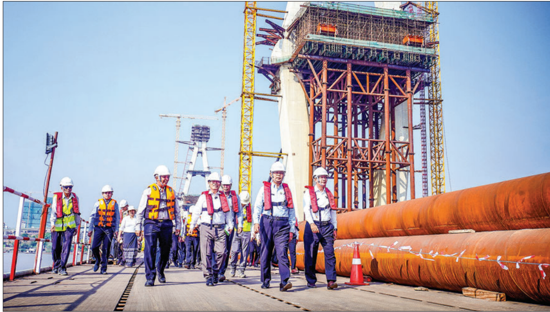
Union Minister for Construction U Myo Thant looks into progress of Myanmar-Korea Friendship Bridge (Dala), in Dala, Yangon Region yesterday.
