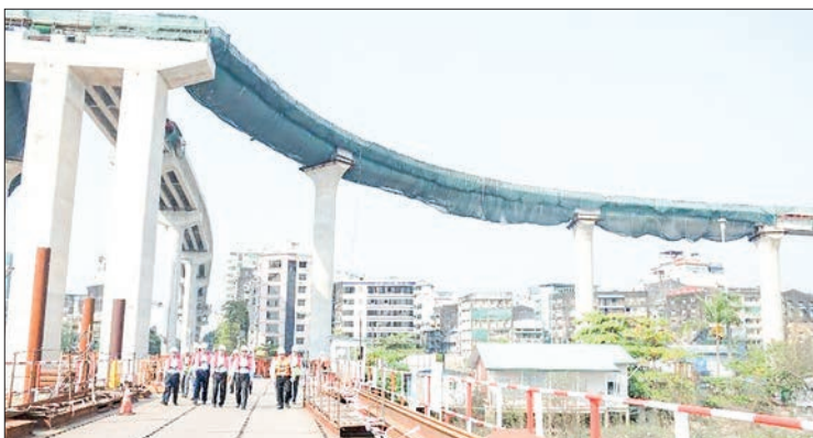
The Union Minister for Construction inspects construction sites of the Myanmar-Korea Friendship Bridge (Dala).
