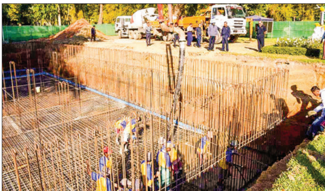
The YCDC vice-chairman and party inspect the construction progress of the underground water reservoir on 1 February.
