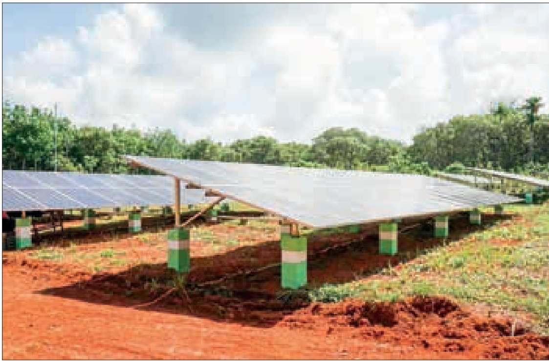
The mini-grid solar system is installed in Aungba Village, Sungebalai Village-tract in Kawthoung Township.
