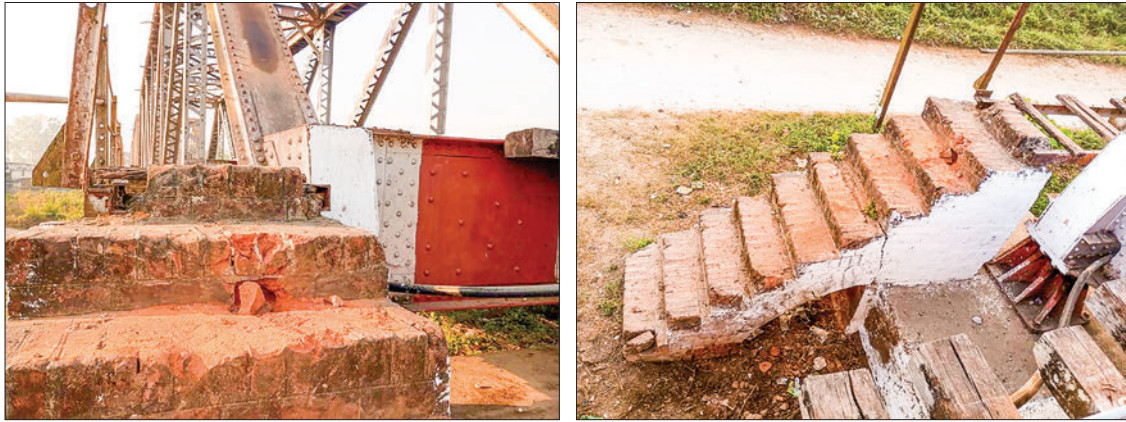
Photos depict the Kabaung Bridge, which is located between Toungoo and Thaungdinegon stations in Toungoo Township, Bago Region, was exploded by terrorists on 12 March.
