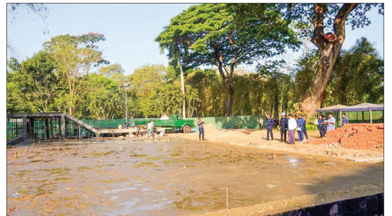
Yangon Mayor U Bo Htay seen inspecting the construction of an underground water tank at People's Square and Public Park on 12 March.
