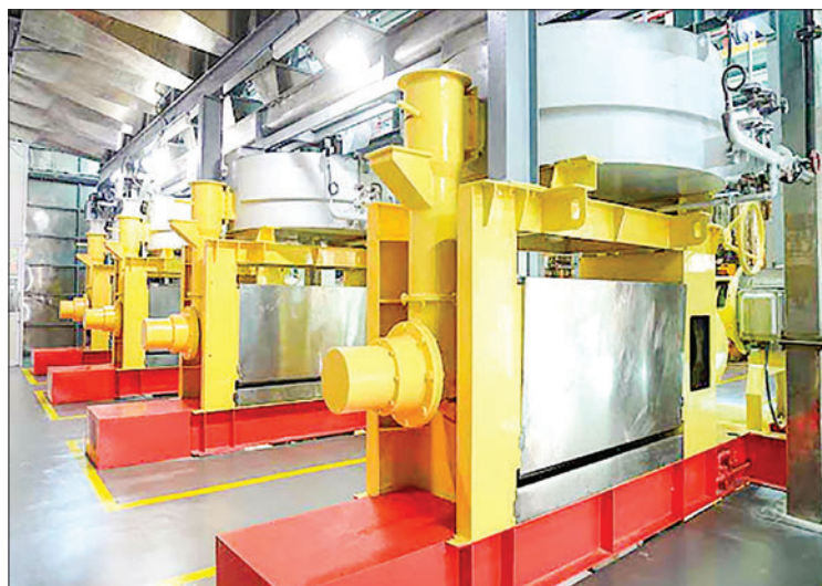
The photo depicts a general view of the local oil refinery.
