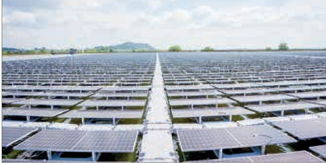
A panoramic view of the floating solar system at the Pahtaw Reservoir in Kyunsu Township, Taninthayi Region.
