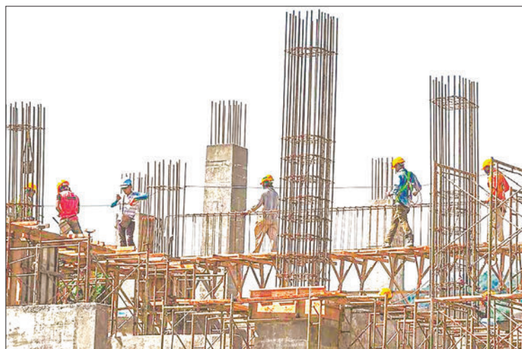
Despite global efforts, the sector's greenhouse gas emissions continue to rise, highlighting the urgent need for innovative solutions to decarbonize construction practices and align with climate goals outlined in the Paris Agreement. PHOTO: PIX FOR REPRESENTATIONAL PURPOSE ONLY/AFP
