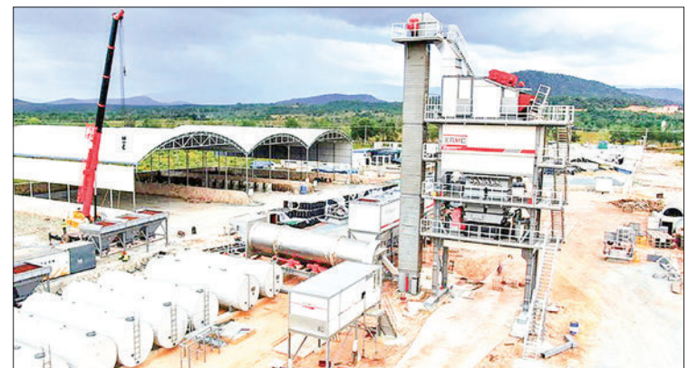
Aerial photo taken on 2 December 2020 shows an asphalt mixing station at the construction site of the first expressway in Cambodia in Koh Kong Province, Cambodia. PHOTO: PIX FOR VISUAL PURPOSE/ LI ZHEN/ XINHUA
