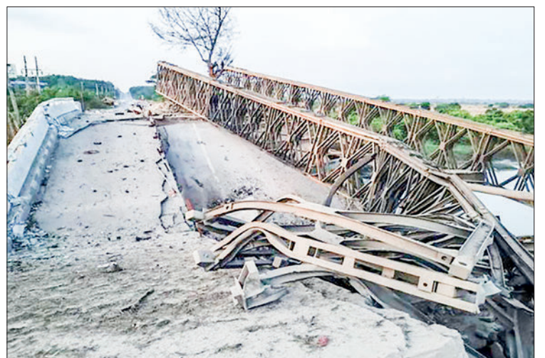
The photo depicts the Kyoneik Bridge, which is connecting between Yangon and Mawlamyine in Thaton Township, Mon State, was exploded by KNLA insurgents and PDF terrorist groups on 11 May 2024.
