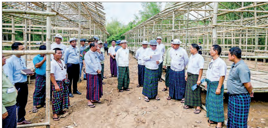
The Kachin State chief minister and officials inspect the construction of bamboo houses for IDPs in Thazinmyaing Village, Myitkyina Township.
