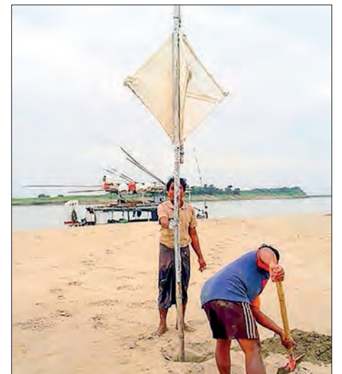
The navigational aid is seen being erected in the Ayeyawady River near Mandalay.
