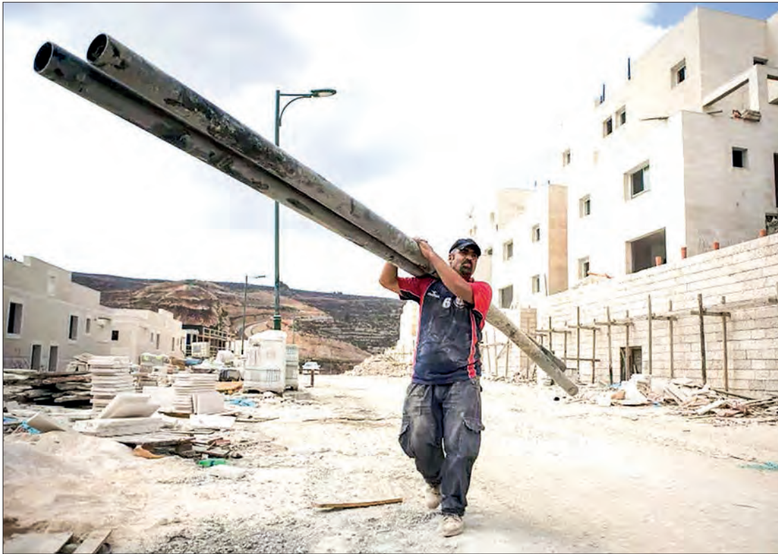
Palestinian labourers work at the site of a new neighborhood in the Jewish settlement of Givat Zeev in the West Bank, north of Jerusalem. PHOTO: MENAHEM KAHANA/AFP/FILE
