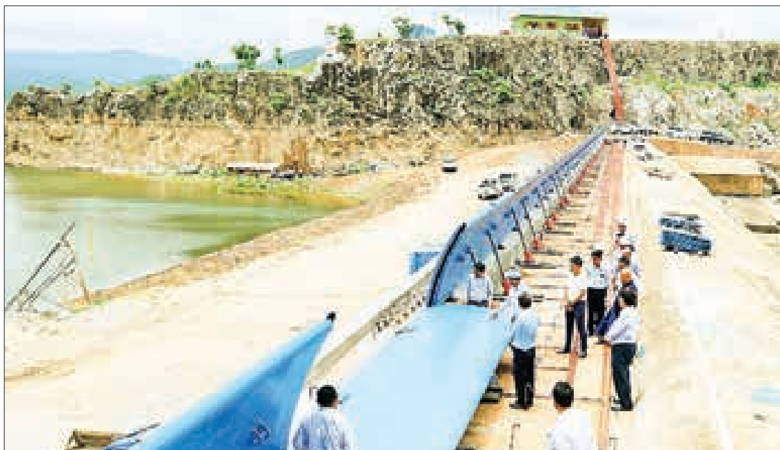
Union Minister for Agriculture, Livestock, and Irrigation U Min Naung and officials are inspecting the installation project of the hydraulic elevator dam at Paunglaung Dam in Zeyathiri Township.
