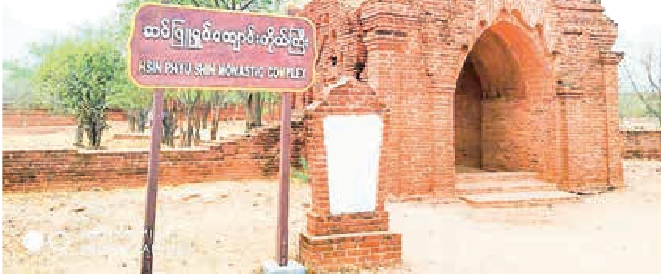
Hsin Phyu Shin monastic complex in the Bagan Ancient Cultural Heritage Zone and restoration work underway.
