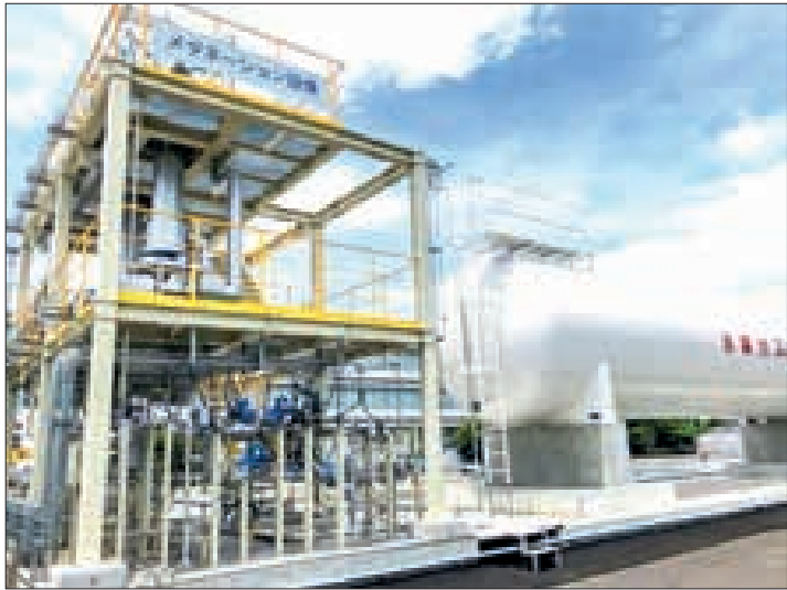
Tokyo Gas Co, Ltd, founded in 1885, is the primary provider of natural gas to the main cities of Tokyo, Kanagawa, Saitama, Chiba, Ibaraki, Tochigi, Gunma, Yamanashi, and Nagano. PHOTO: PIX FOR VISUAL PURPOSE/TOKYO GAS
