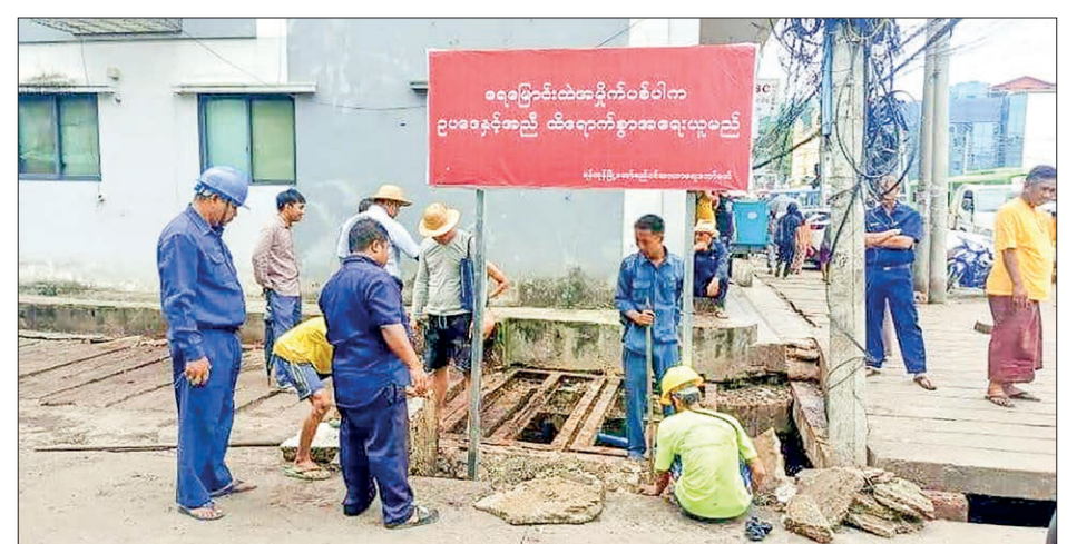
Erecting notice signages for the development of water flow in Yangon City.
