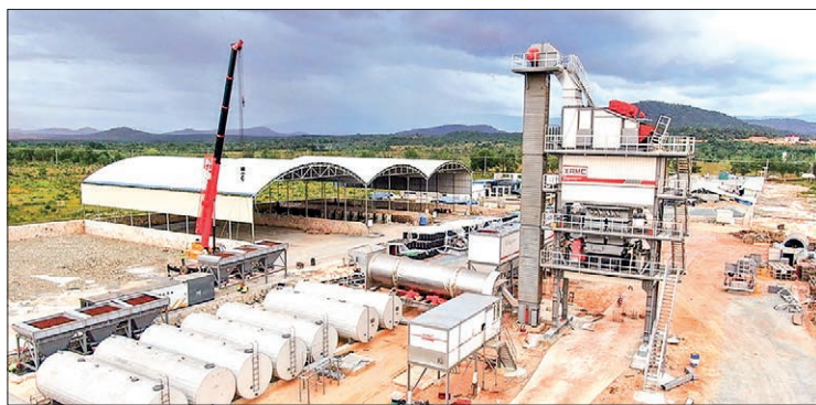
Aerial photo taken on 2 December 2020 shows an asphalt mixing station at the construction site of the first expressway in Cambodia in Koh Kong Province, Cambodia. PHOTO: LI ZHEN/XINHUA
