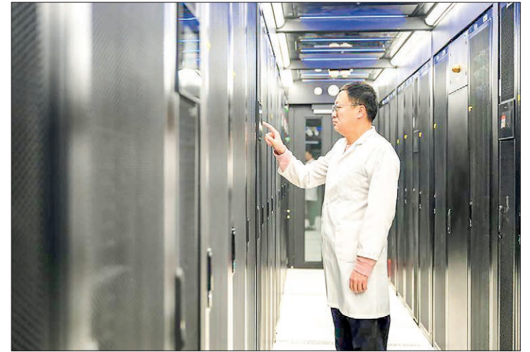
A staff member checks equipment at a data centre of China Mobile in Horinger, Hohhot City, north China's Inner Mongolia, 28 November 2023. PHOTO: XINHUA
